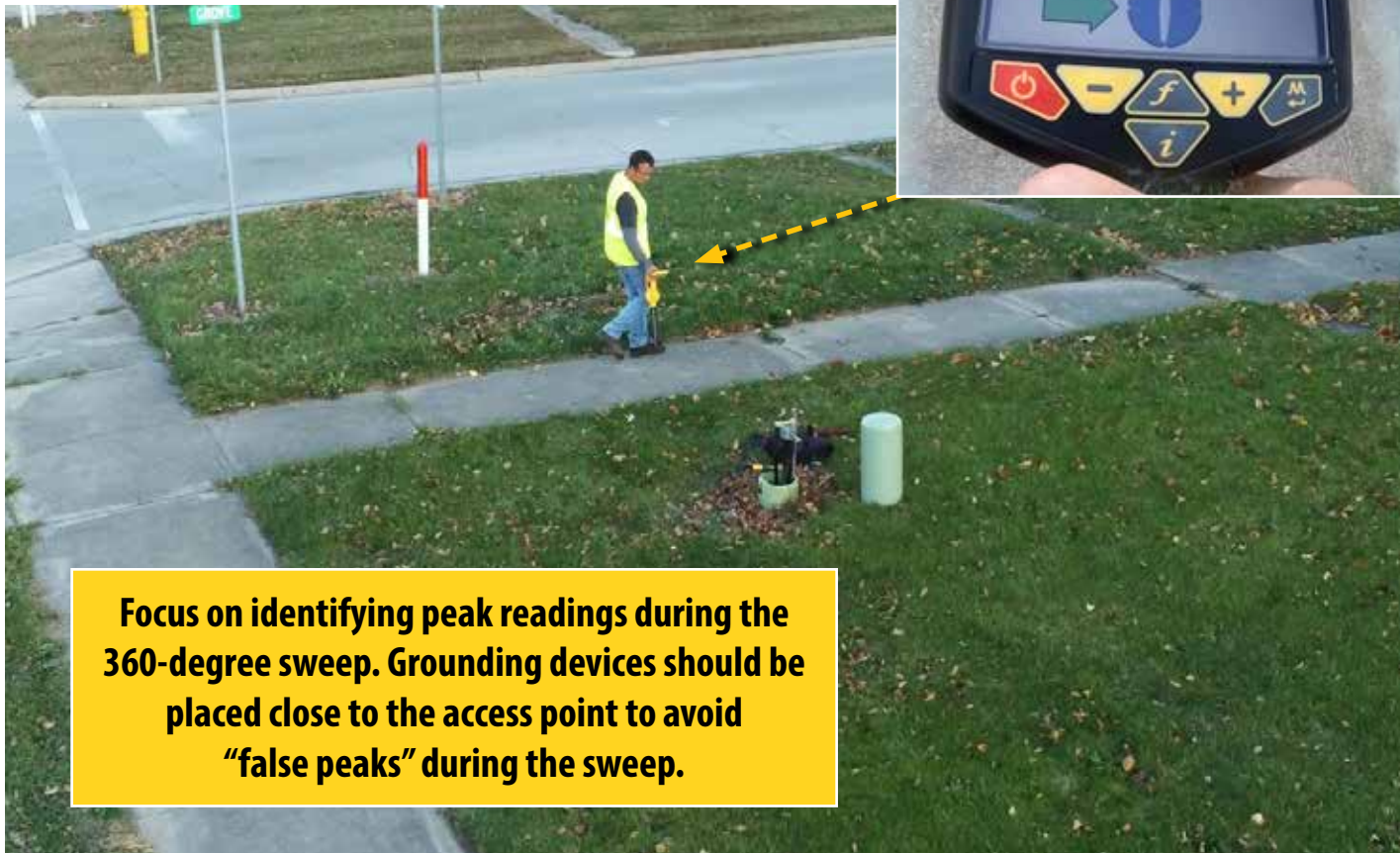
Figure 42: The operator adjusts how the receiver is being oriented as he walks around the access point.
