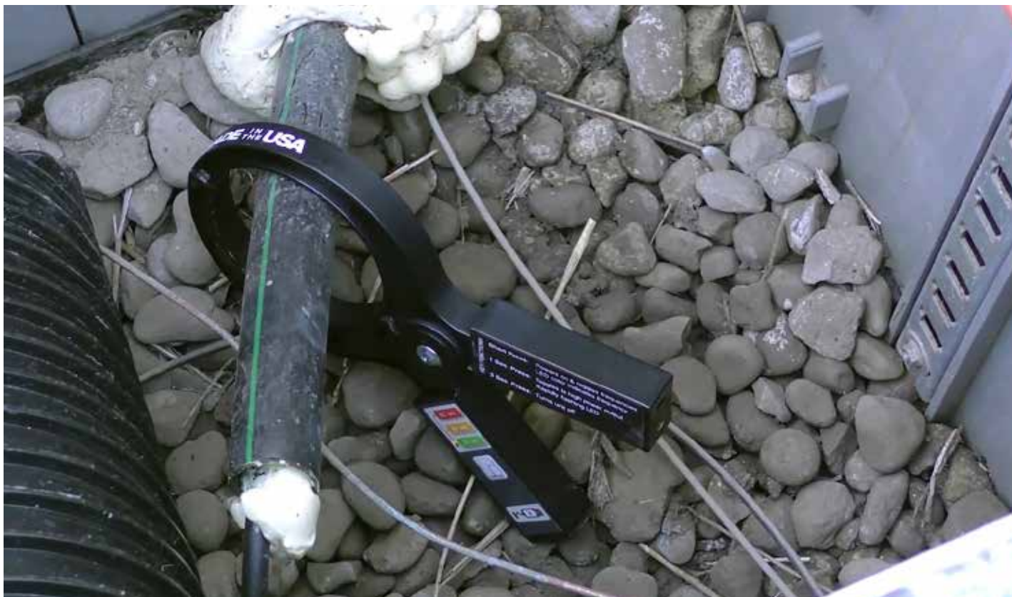
Figure 21: The use of the inductive coupler produces current that flows not only on the metal pipe or cable, but also through the earth.
