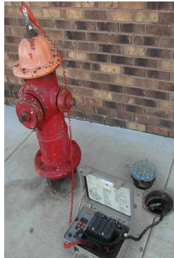
Figure 16: A connection to a water hydrant and a ground using a hydrant valve box.
