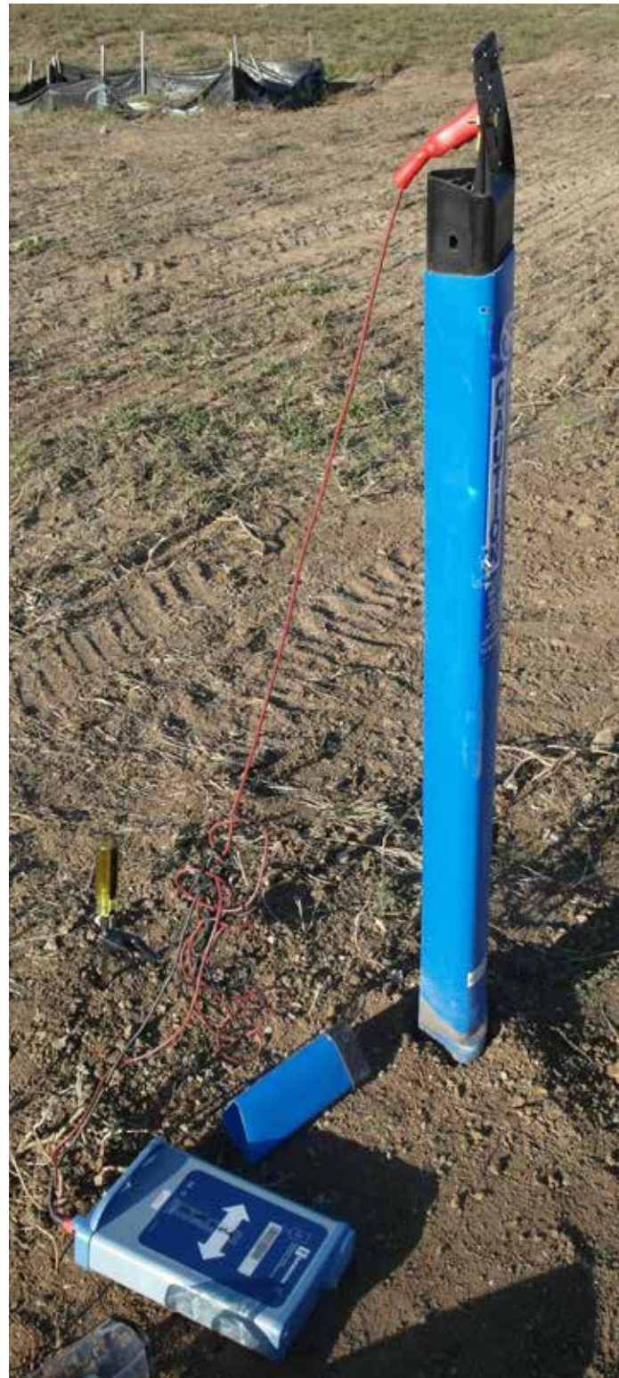
Figure 17: Connections to a tracer wire for a plastic water main and a screwdriver.
