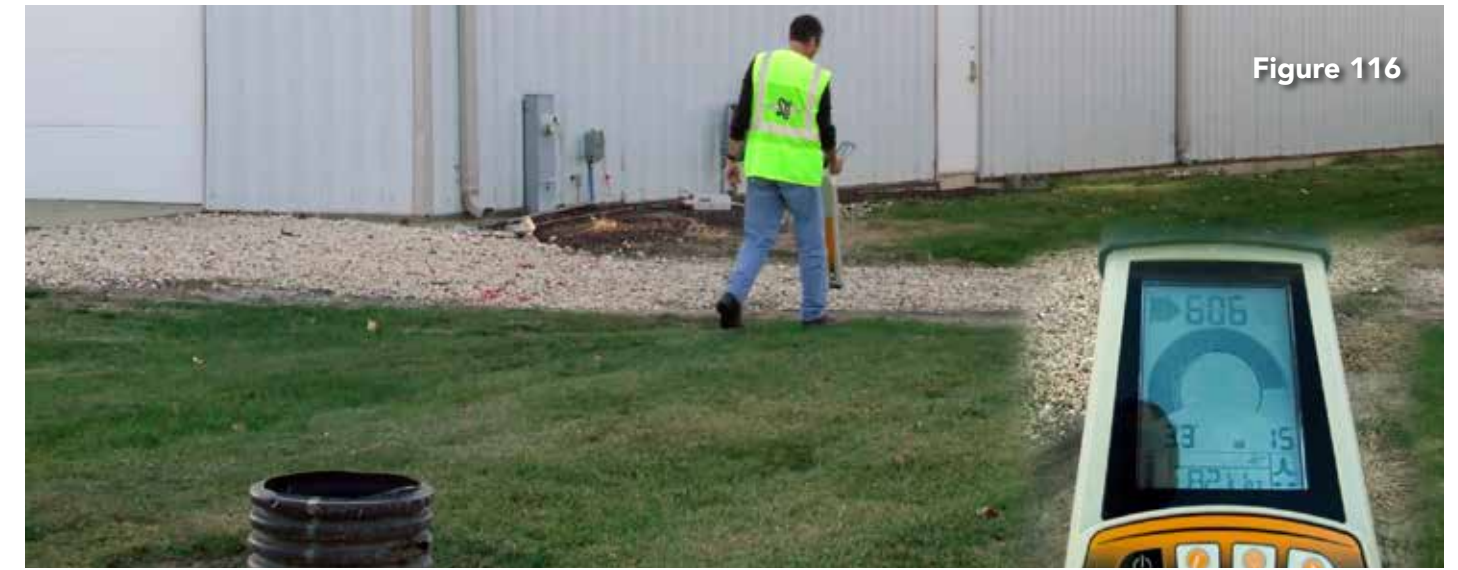
Looking at the red paint on the ground and performing a trace back to the starting point reveals the signal is not on the electric line (Figures 116-117). A turn in the phone drop is indicated once the peak reading decreases significantly (Figure 117). Upon turning, the trace is directed toward the telephone box (Figure 118).
