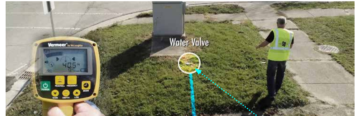
Figure 63: Continuing to locate the cable TV feeder line now quite a few feet west of the water main.
